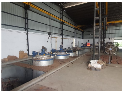
HEAT TREATMENT SHOP
